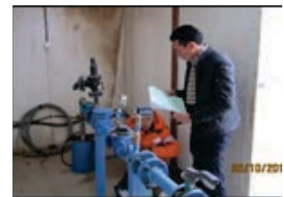
4. Equipped supply well
